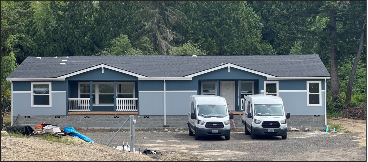
One of two transitional houses being set up by Court Services building
